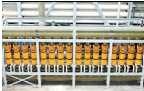
Figure 5: Isobaric Energy Recovery System manufactured by Energy Recovery Incorporated and used at PSDP
