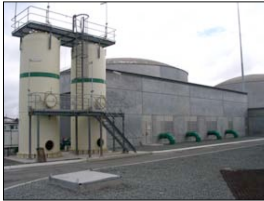
Figure 4: Concrete Walls and Acoustically Treated Louvres house the Drinking Water Pumps.
